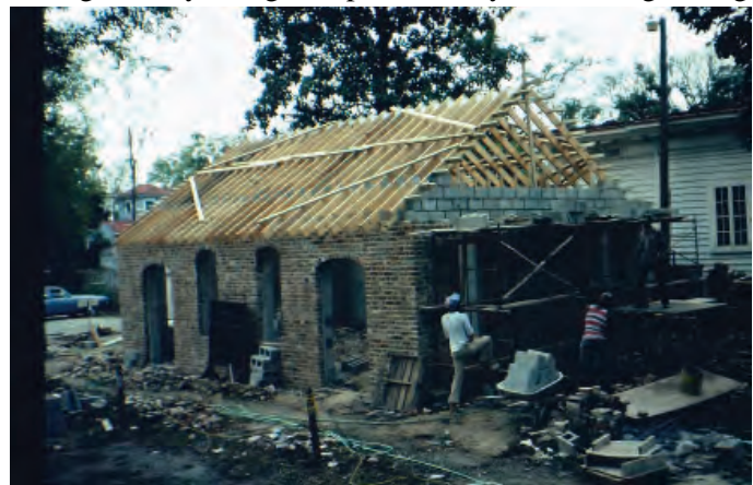
Haslen Dependency, ca. 1760-1770, 513 Broad Street, located behind the Attmore-Oliver House. Moved to this site and reconstructed 1980-1986.
